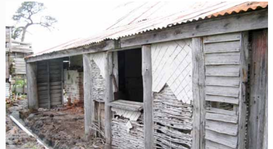
An 1840s farm cottage in an advanced state of deterioration
