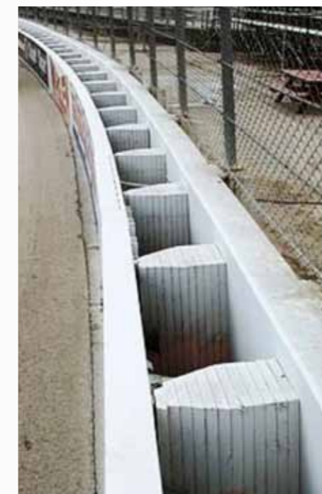
A SAFER barrier installed at the Milwaukee Mile. Photo courtesy of Wikipedia.
