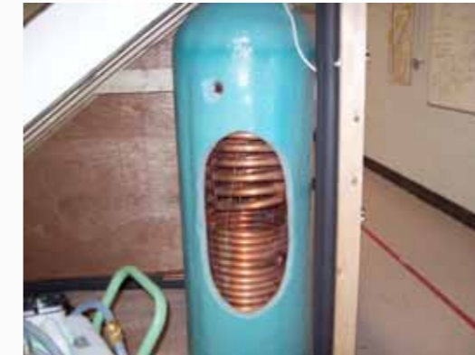
Figure 19: Internal cylinder operation having two heat exchange coils (the inside one is for a closed glycol system from rooftop solar panels, the other is for a sealed domestic hot water exchange coil)
