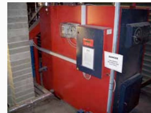
Figure 35: 240 kW KSM wood chip boiler installed at Wasing Estate
