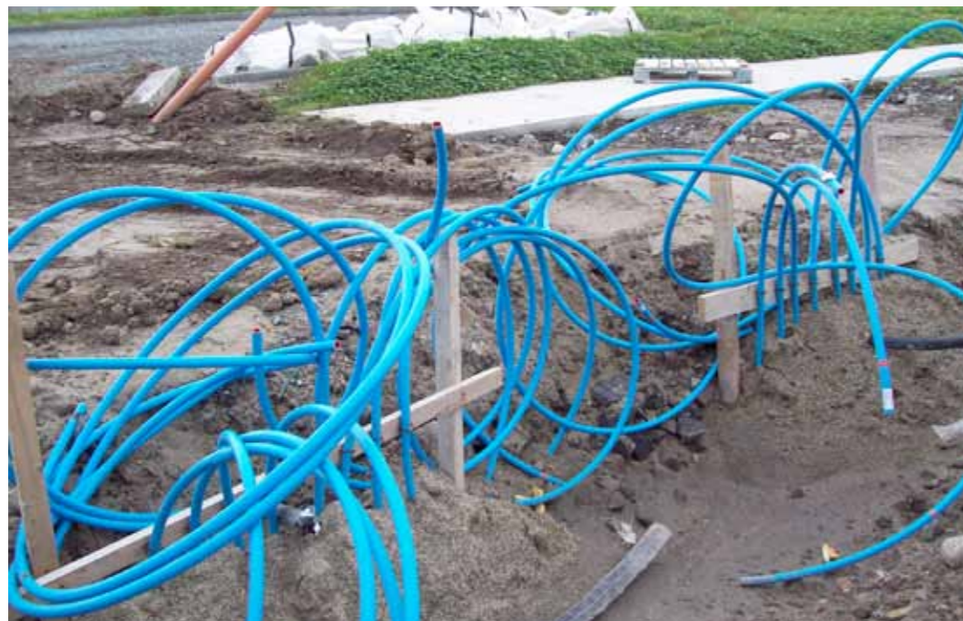
Figure 6: Flow and return collector poly pipe lines from lawn area (note: the lines are not yet connected to the manifolds).
