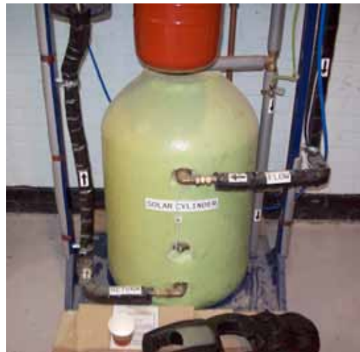
Figure 15: Solar heat exchange cylinder
