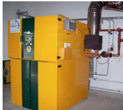
Figure 4: One of the two 150 kW KWB Powerfire willow chip boilers
