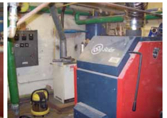
Figure 31: The 38 kW KSM 'Stoker' biomass boiler installed in the basement of the school (note the old gas unit in the background)
