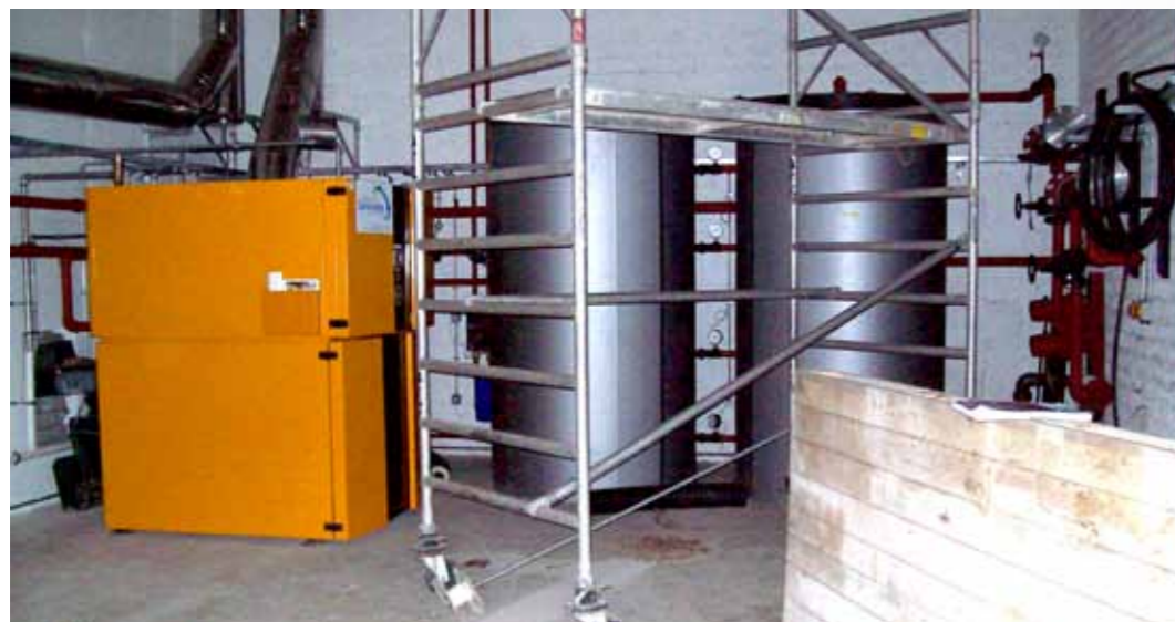
Figure 5: Second of the two KWB Powerfire boilers, with well insulated buffer storage tanks
