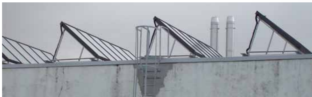
Figure 8: Solar panels on the roof at Údarás Industrial Park (the two flues in rear of picture were connected to the biomass boilers in the plant room)
