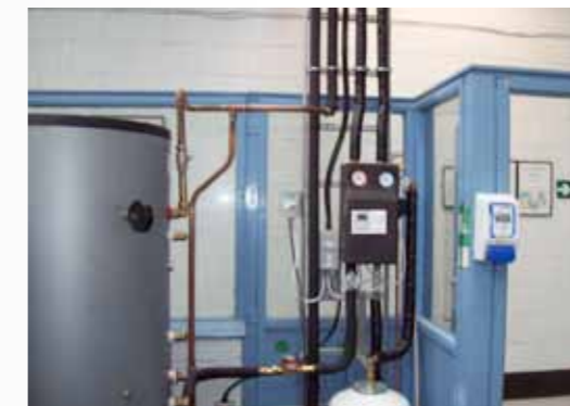
Figure 21: The large, fully functional solar unit installed in the FAS plumbing workshop (this unit had solar panels fitted on the roof and monitoring gauges so apprentices could see the heat process in operation)
