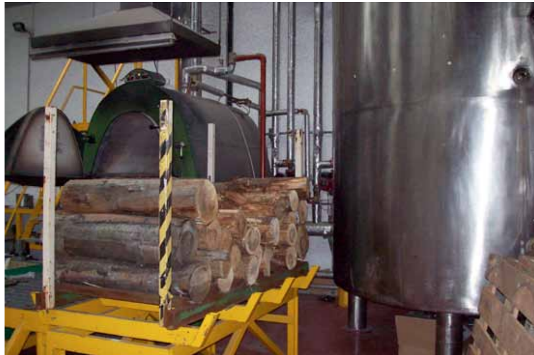
Figure 1: Herit gasifying boiler and buffer storage tank at Údarás Industrial Park
