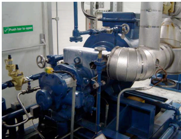
CO 2 / Ammonia cascade system Star Refrigeration ASDA Distribution Centre Glasgow
