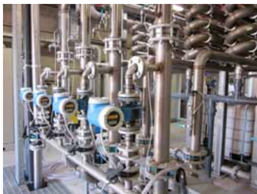
MBR treatment plant
