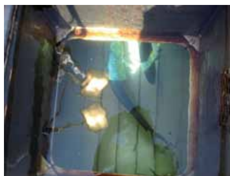
Figure 16b: Lights over the tank
