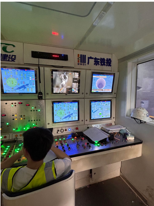
Figure 7. Control room on TBM constructing the Guangzhou to Zhaoqing high speed railway, Guangdong, China
