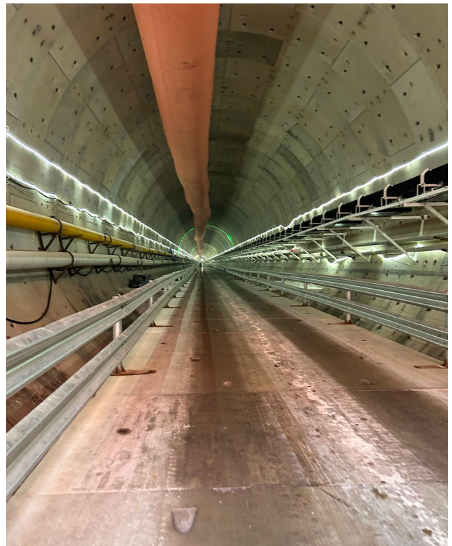
Figure 1. Segment lined tunnel under construction for the Guangzhou to Zhaoqing high speed railway, Guangdong, China.
