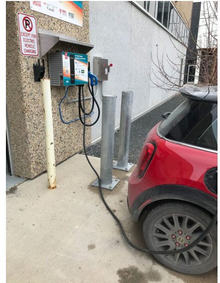
Figure 58. RRC Polytechnic, MotiveLab eV charging point
