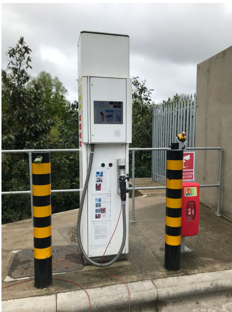
Figure 15. Metroline Perivale workshop H2 refuelling bowser
