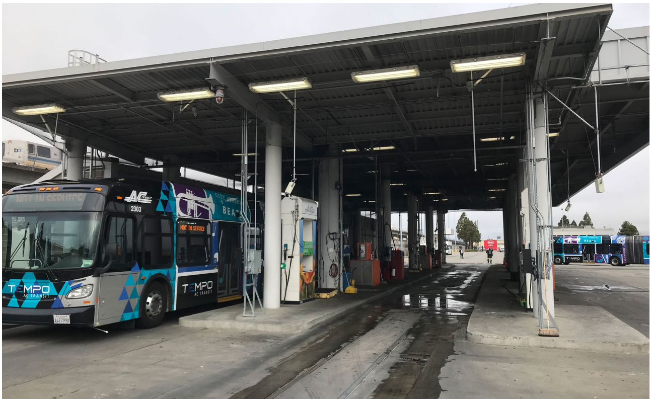
Figure 4. AC Transit Training Maintenance Depot Hydrogen Re-Fuelling Station
