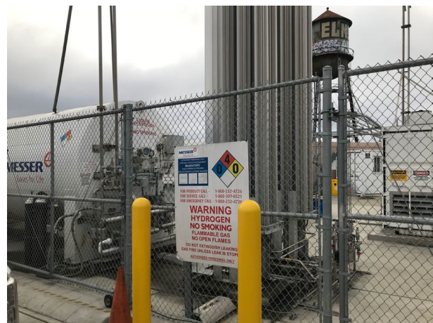
Figure 3. AC Transit Training Maintenance Depot Hydrogen Storage Facility
