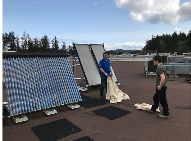
Figure 29. James Smyth Plumbing teacher & vocational education plumbing student (Vacuum solar arrays)
