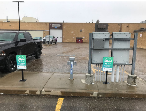
Figure 48. EV charger converted from heating station
