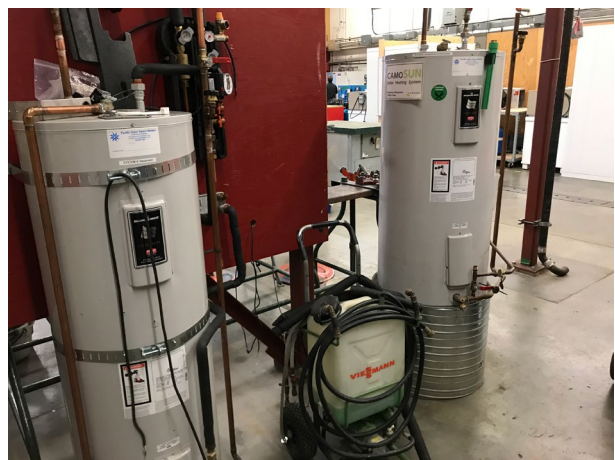
Figure 31. Camosun College Plumbing Centre – Hot water lab
