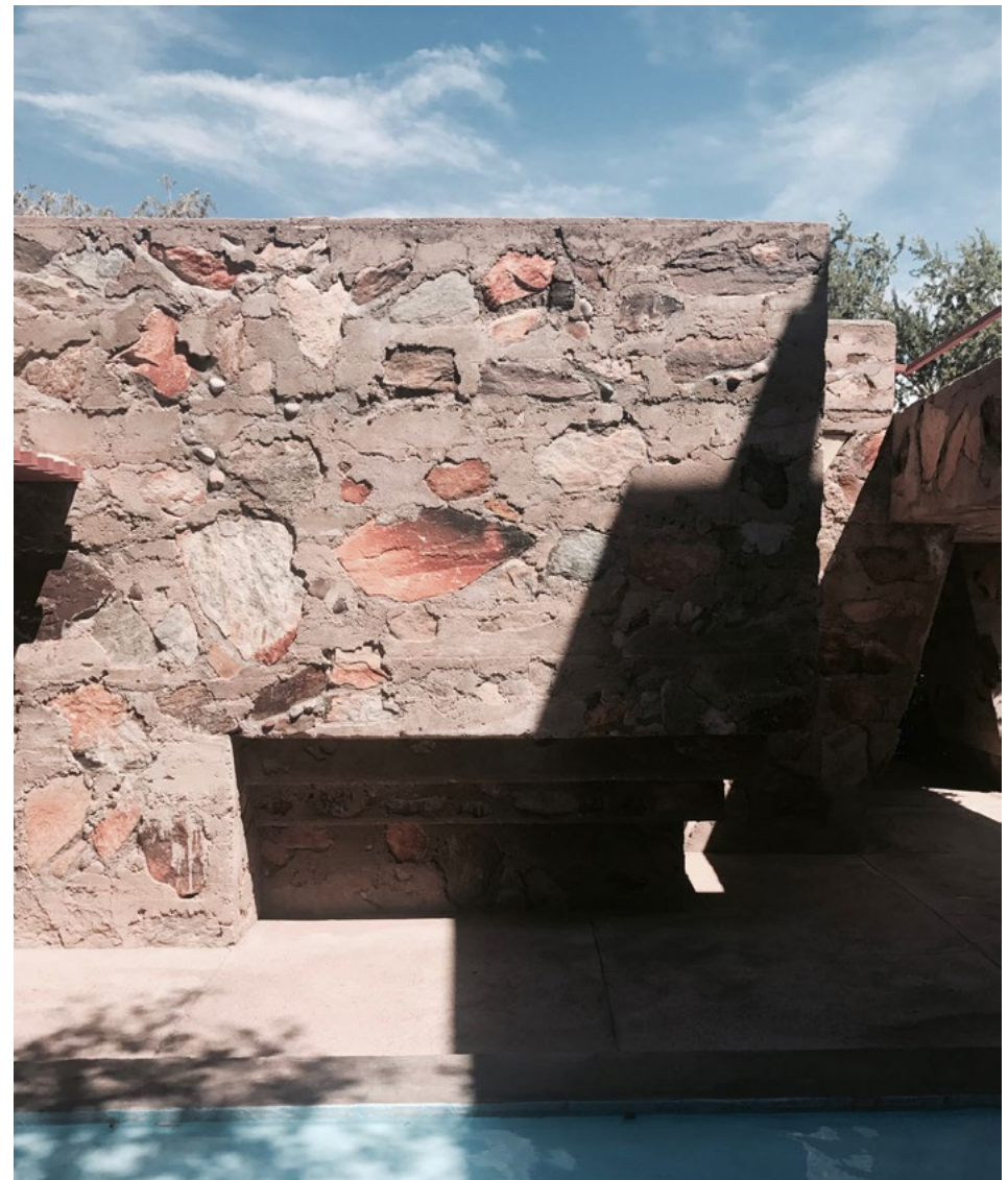
The rock masonry made from local stone and cement at Taliesin West.
