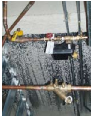
Specialised pipe fittings St. Joseph's Hospital Ann Arbor
