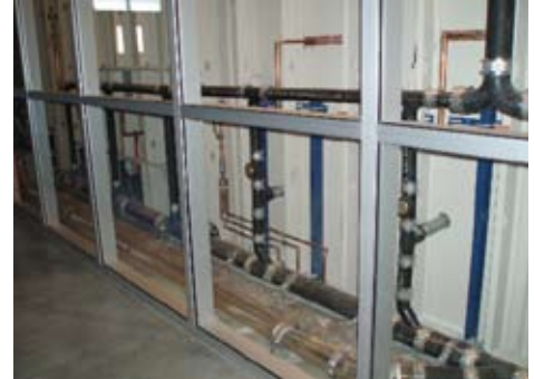
Exposed pipes and glass pipes to examine installation and flow of liquid
