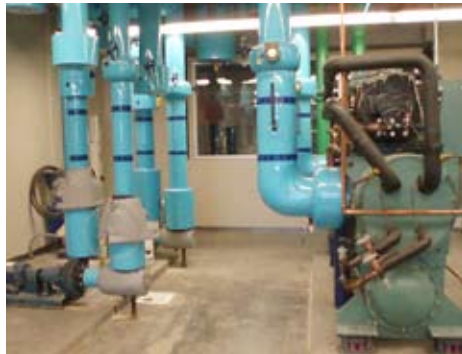
Chiller room installations
