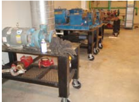
Pump training facilities
