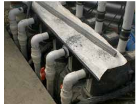
Array of pumps in parallel
