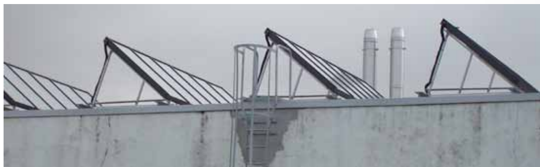
Figure 8: Solar panels on the roof at Údarás Industrial Park (the two flues in rear of picture were connected to the biomass boilers in the plant room)
