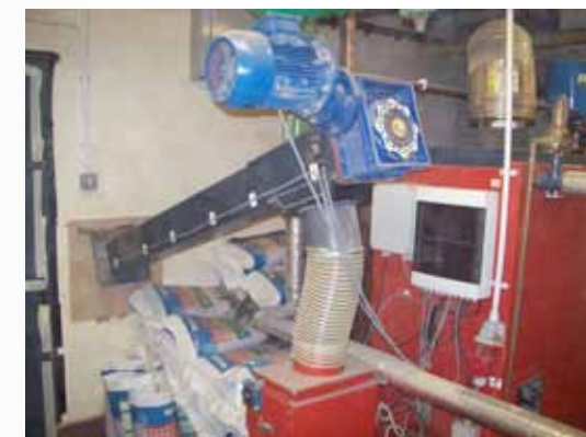
Figure 30: Feed auger for pellets from old coal store in basement of school (also pictured are some spare bags of pellets)
