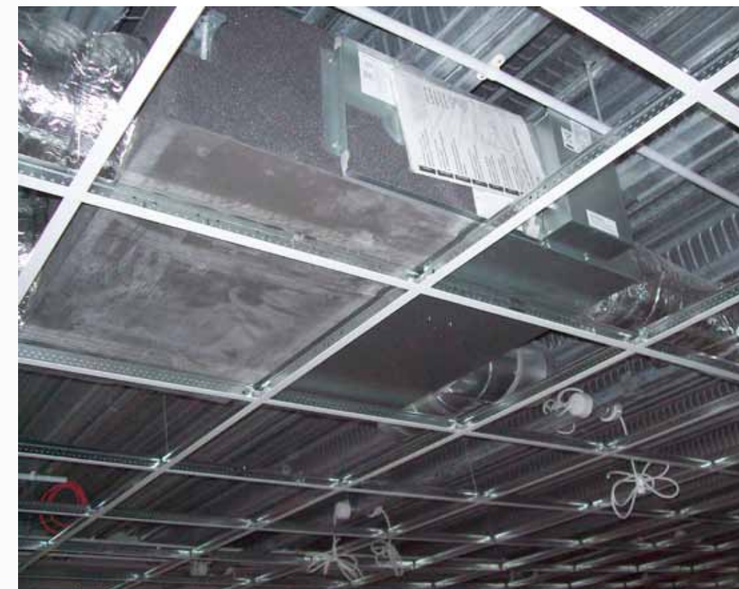
Figure 9: The air handle unit in the ceiling area of a crèche on the ground floor building of Údarás Industrial Park
