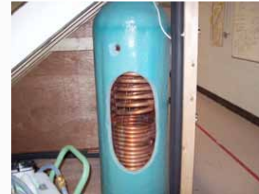
Figure 19: Internal cylinder operation having two heat exchange coils (the inside one is for a closed glycol system from rooftop solar panels, the other is for a sealed domestic hot water exchange coil)
