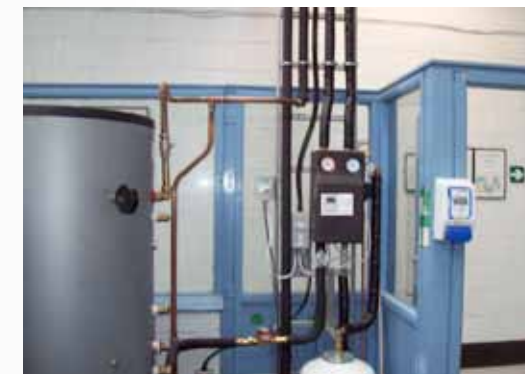
Figure 21: The large, fully functional solar unit installed in the FAS plumbing workshop (this unit had solar panels fitted on the roof and monitoring gauges so apprentices could see the heat process in operation)
