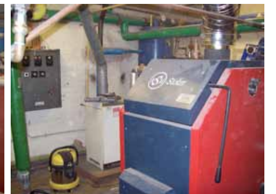
Figure 31: The 38 kW KSM 'Stoker' biomass boiler installed in the basement of the school (note the old gas unit in the background)
