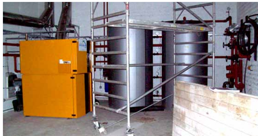
Figure 5: Second of the two KWB Powerfire boilers, with well insulated buffer storage tanks
