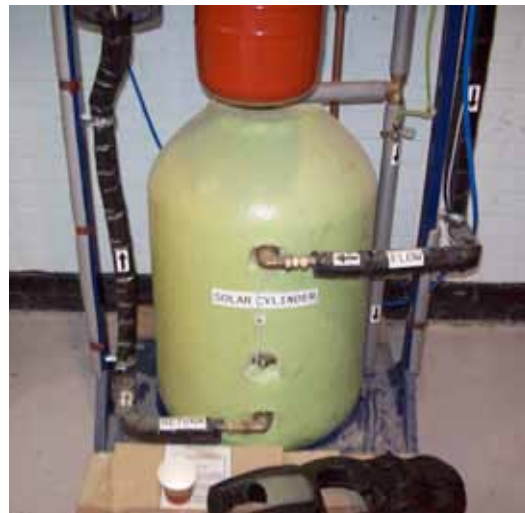
Figure 15: Solar heat exchange cylinder
