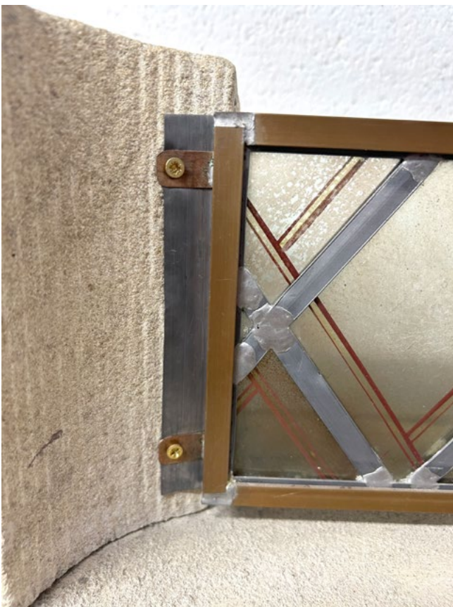
Figure 16. This close-up shows the lead flashing and copper tab fixing system used to secure the frame to the face of the masonry.
