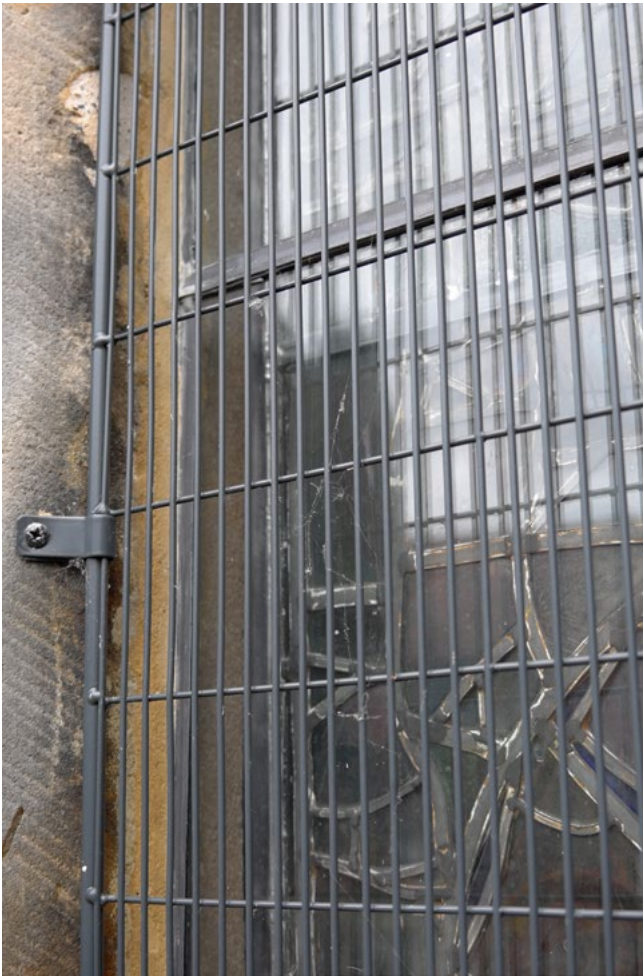
Figure 24. Detail of powder coated protective screens over environmental protective glazing at All Saints North Street, York. Environmental protective glazing by Barley Studios.
