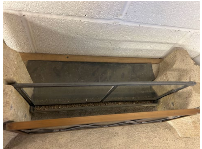
Figure 17. a top down view of the internally ventilated EPG model. Including the lead upstand filled with pebbles and the lead flashing positioned out and down the external face of the masonry.
