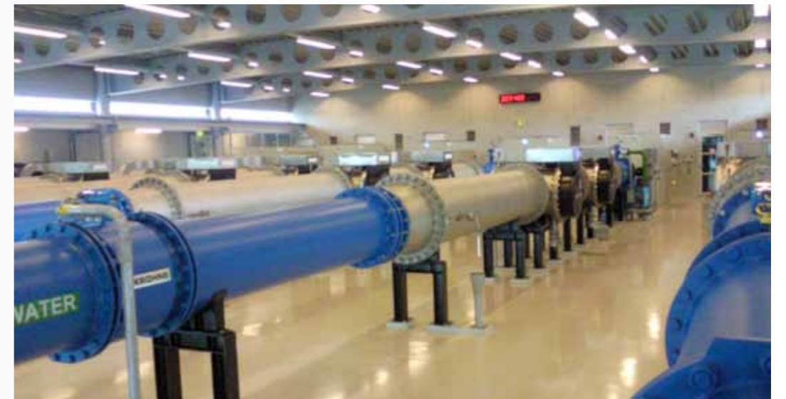
Ultraviolet room, Evides Industriewater
