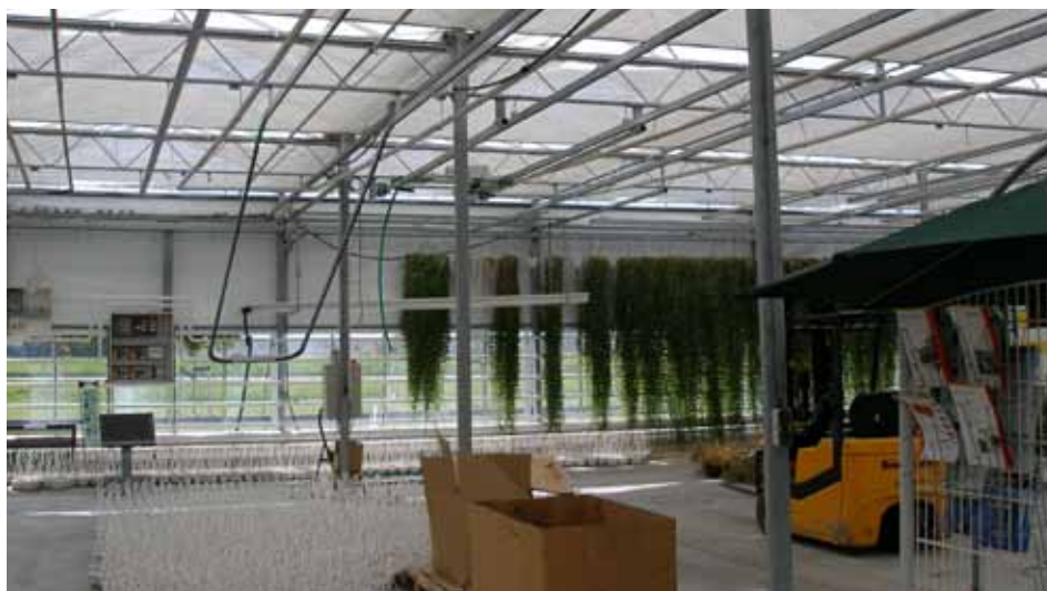
Hoisting system for hanging basket crop support
