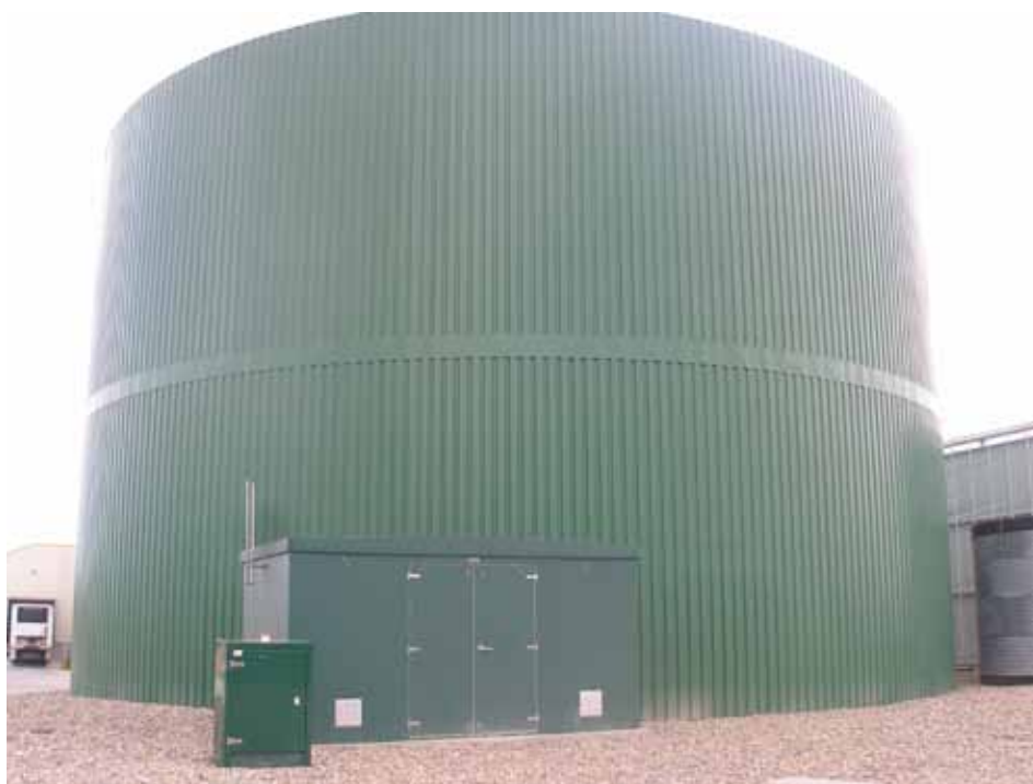
Hot water buffer tank
