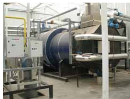
Hot water boiler
