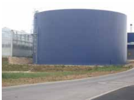
Heat buffer tank
