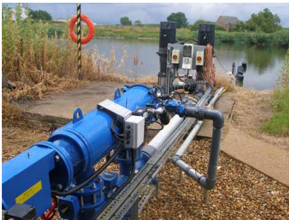
Water filtration system
