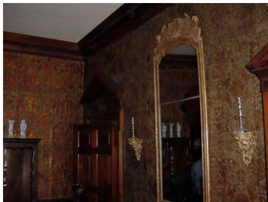
Existing leather wall covering internal walls Governors Palace in the upstairs middle room.
