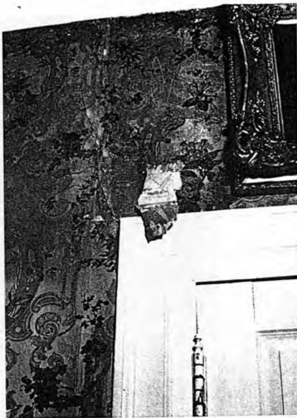
FIG. 2 Parlor paper before treatment. Detached flap exposing underlying paper. Tears in paper along plaster cracks evident in area left of flap. Waterstaining along top edge.
